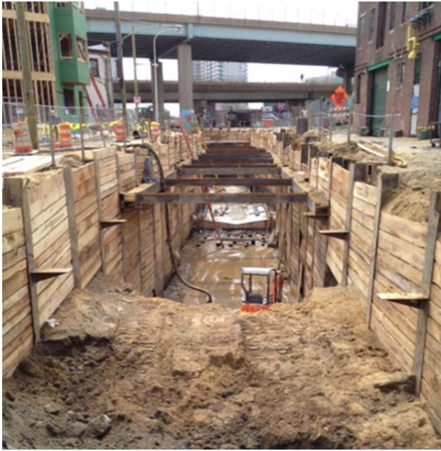
FIGURE 2. Construction activities for the Northern Liberties SFR Project showing an open cut installation of a box sewer.
